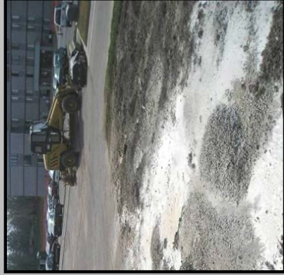
Wash out of solids/liquids
