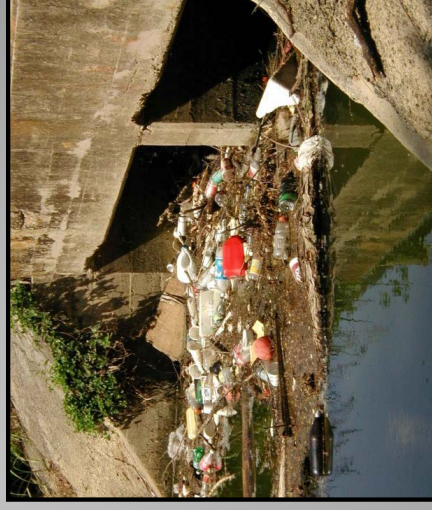
Trash and debris
